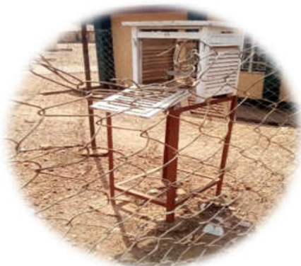
FIGURE 1: Abandon & dilapidated School Meteorological Station at GSSK
